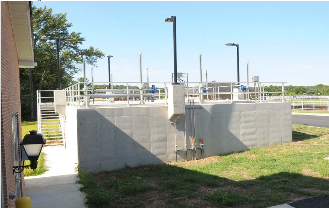
Stormflow Diversion Chamber
