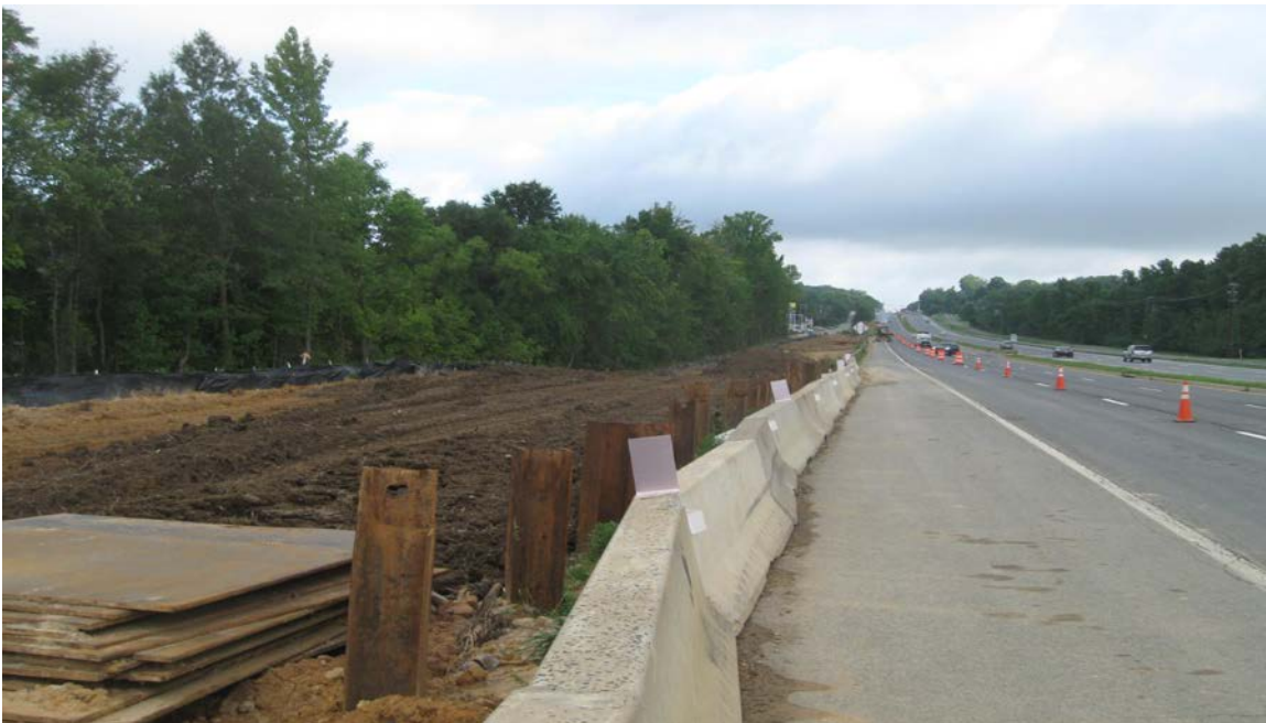
Looking north on MD 210 from Swan Creek Road – Top soil placement after pipe installation
