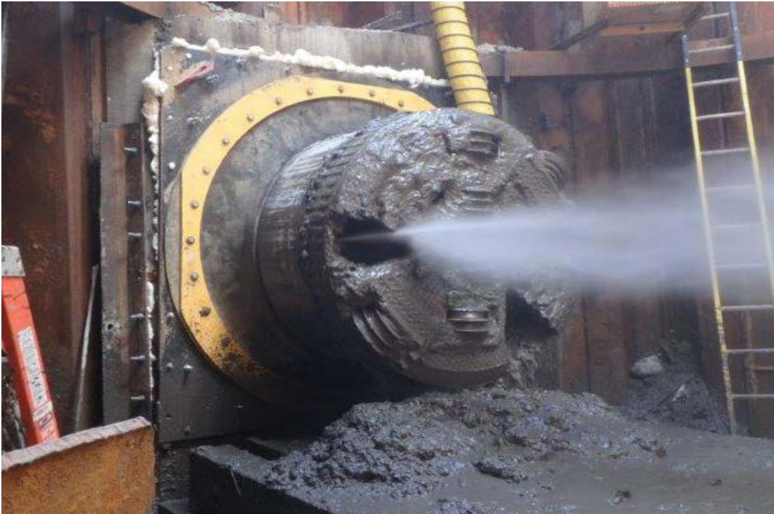
Hole thru of Micro Tunnel Boring Machine on Tunnel 6 (From east side of MD 210 to West side)
