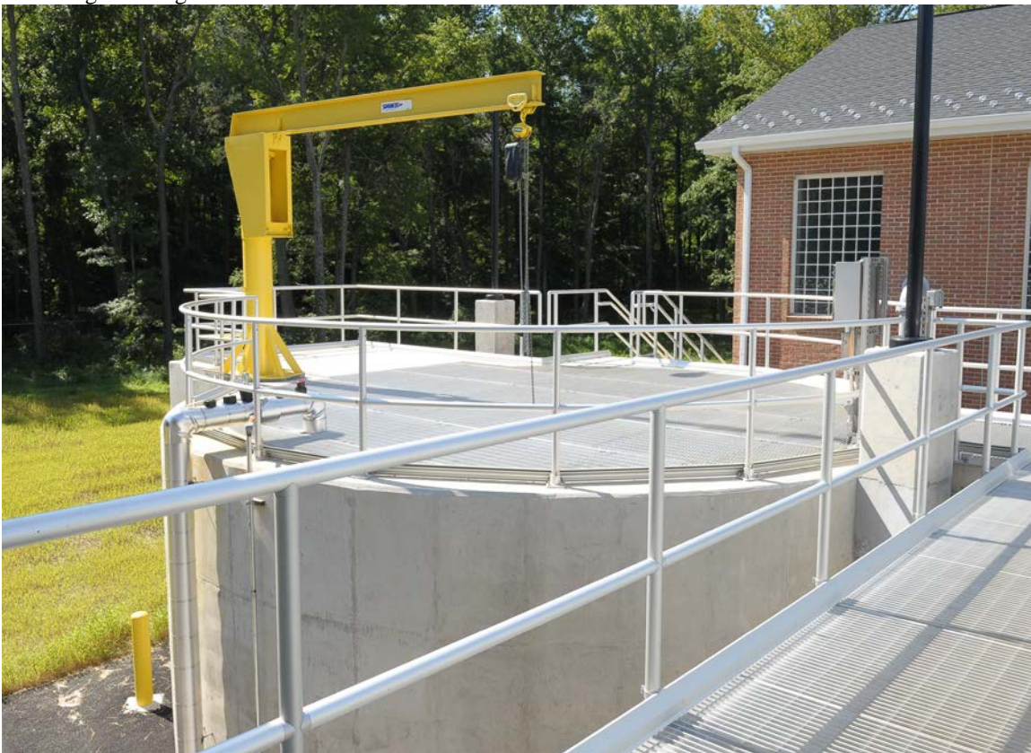
Grit Removal Unit
