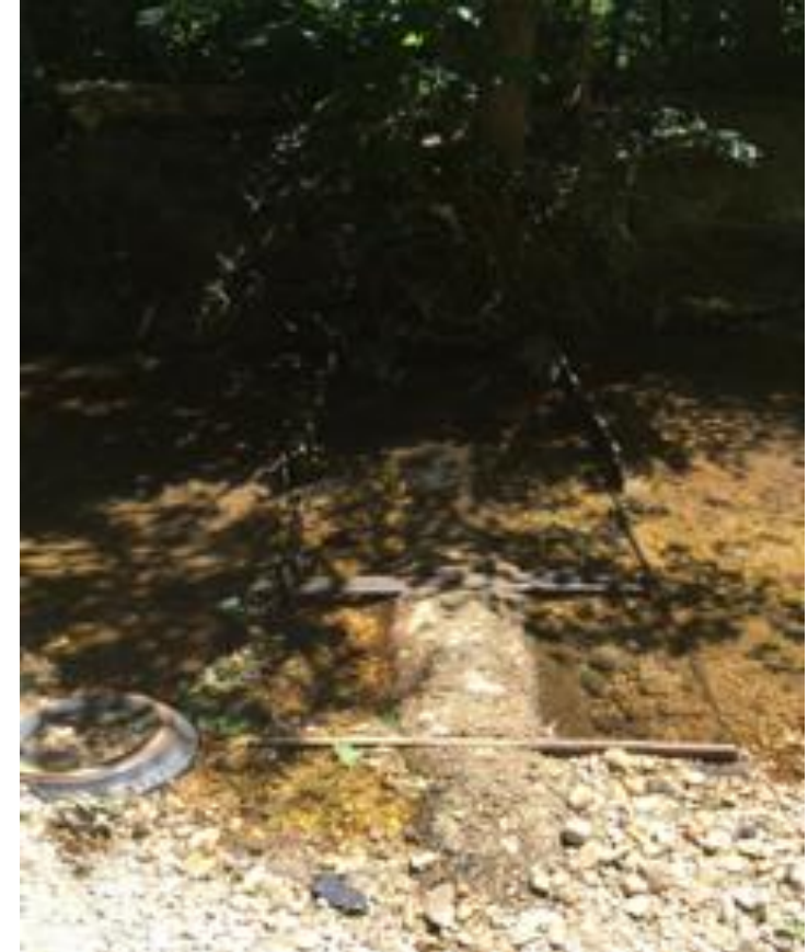
An exposed sewer pipe in a forest
