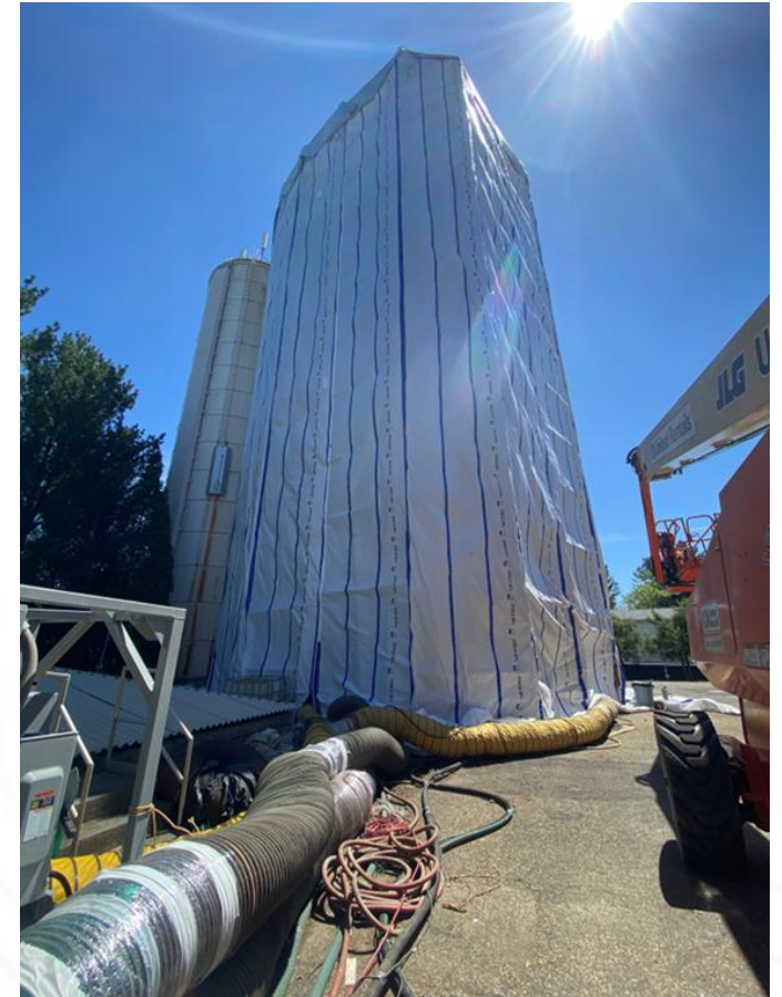
A complete class 2-A containment system
