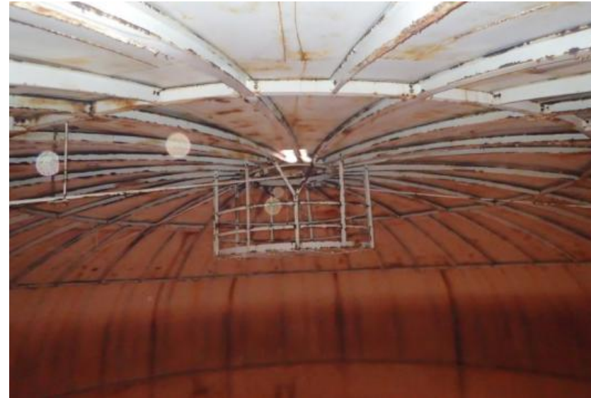
◀ Corrosion on tank roof
