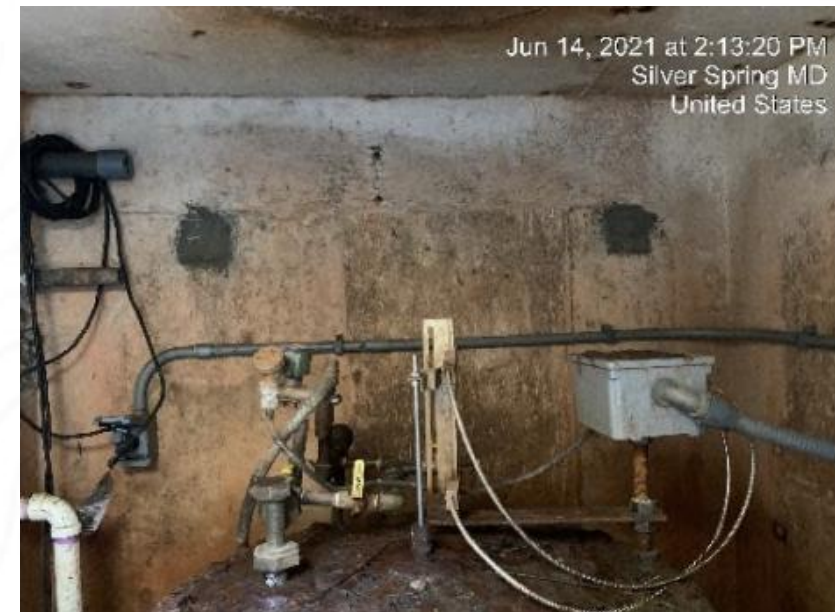
◀ Outdated equipment in altitude valve vault
