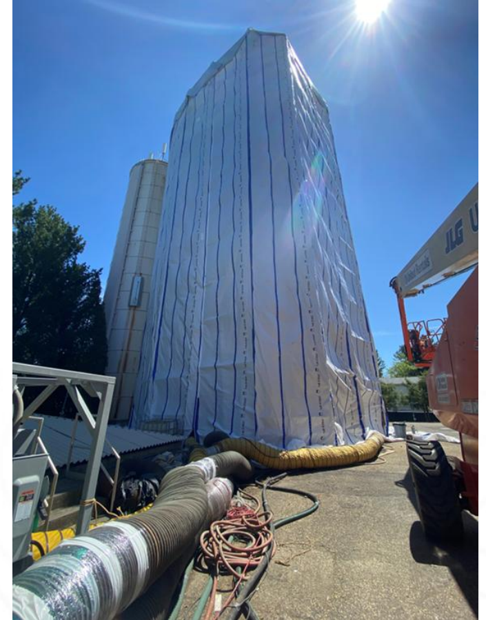
A complete class 2-A containment system
