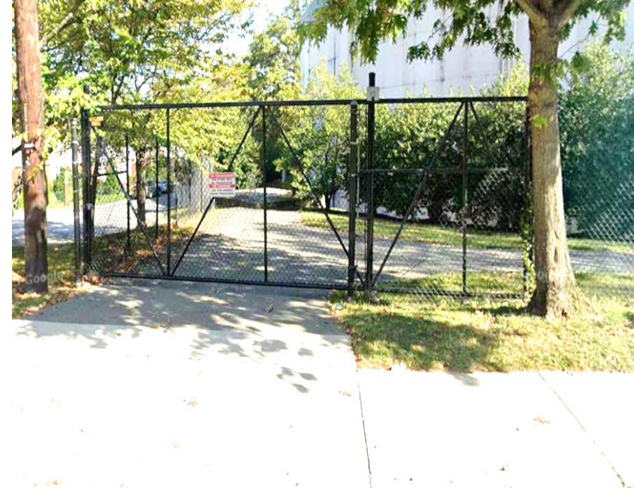
An example of vinyl security fencing at a WSSC Water facility in Wheaton.
